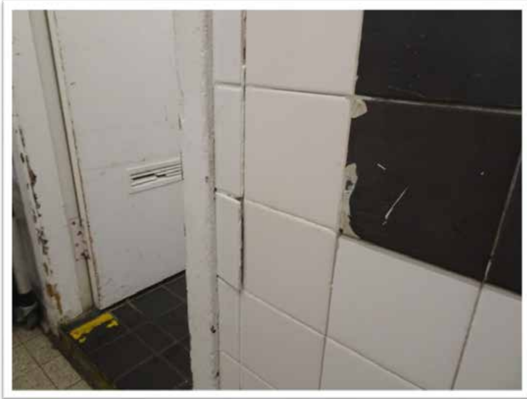
Unclean tiles in kitchen
